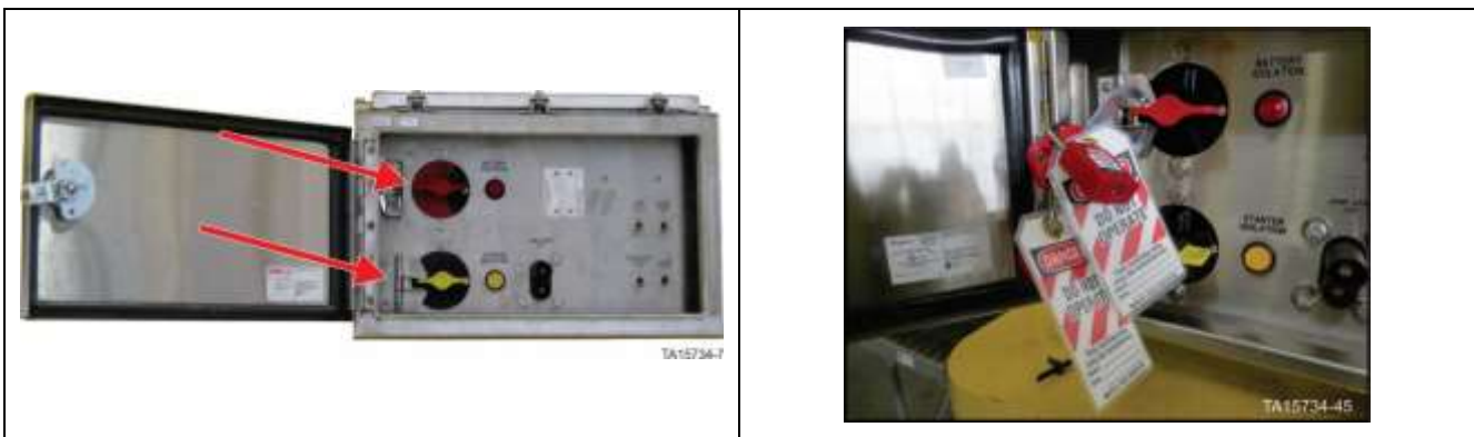
Figure 4. Isolation and control switch assembly
